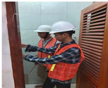
Gambar 4 Perapian Ruang Control
