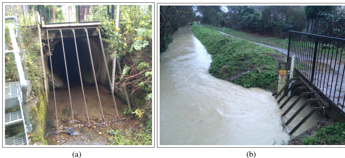
Figure 5.2 Gough Way culvert entrance with (a) base flow and (b) calibration event on July 12th 2012 (courtesy of Keith Glover)
