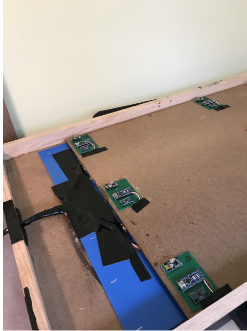
Figure 4.5: We run all the wiring for powering the sensors outside of the sensor box to the batteries.
