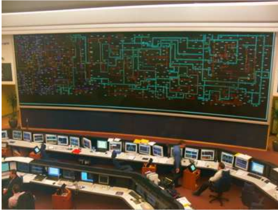
Figure 1-1. National Grid Electricity Control Centre, the voltage switching takes place on the desk directly in front of the transmission network map.
