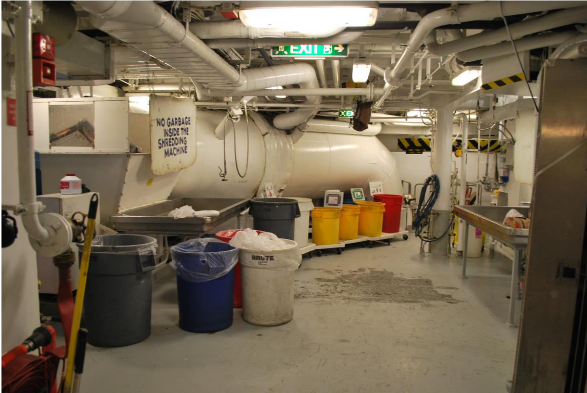
Figure 3. The waste handling room on board Brilliance of the Seas (6.6.2015). Information on which kind of waste belongs to which barrel is visibly demonstrated for the crew members. (Photograph: Irina Svaetichn)
