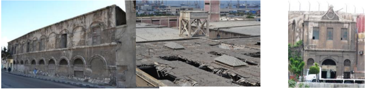
Figure 17: Pictures of Makbas 45 side elevation, roof and on the right the remaining remarkable façade facing the canal (Source: authors, 2012).
