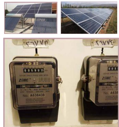
Figure 5 Net metering is a RE incentive, and install SWH Source: ("The National Renewable Energy Action Plan for the Republic of Lebanon", 2016)
