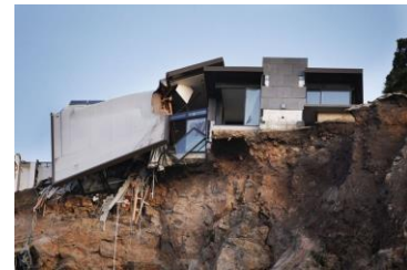
Fig.3: Construction problem on difficult topography
