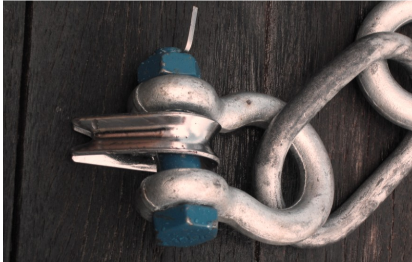
Figure 3: The thimble where the 14 mm Meteor line is missing causing the preliminary loss of 2 km of the instrument line.
