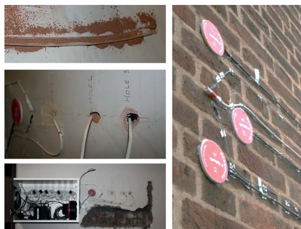
Fig. 2. Installation of the hobo sensors in the wall. Anti-clockwise from top left: hobo sensor in half tube filled with brick dust, packing brick dust into diagonal holes in wall, measurement equipment on internal surface with some plaster removed, measurement equipment on external surface.
