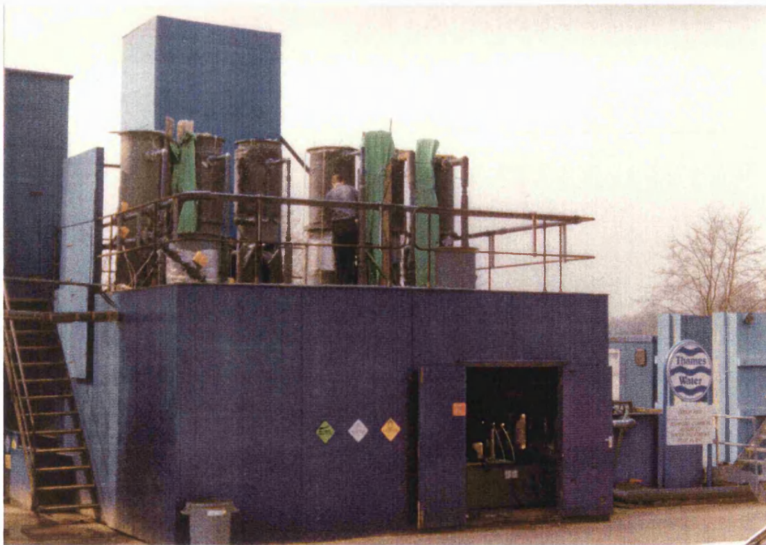
Figure 3.4. The pilot plant in 1992, with deeper filters and ozone contactors enclosed for weather protection.
