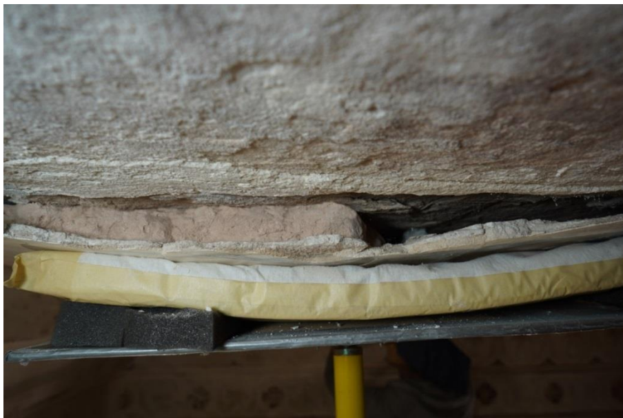
Fig.5: Delaminated area partially filled with grout G, showing good adhesion, with multi-layer absorbent press (©The Courtauld Institute of Art, 2016)
