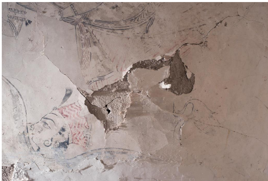
Fig.1: Unstable deformed delamination on the ceiling of the Loggia of the Hadi Rani Mahal (Ahhichatragarh fort and palace complex of Nagaur, India); raking light (©The Courtauld Institute of Art, 2015)
