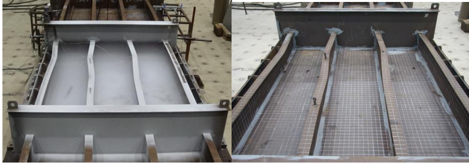
(b) Status after reaching the ultimate strength at the temperature -80^{\circ}\text{C} .
