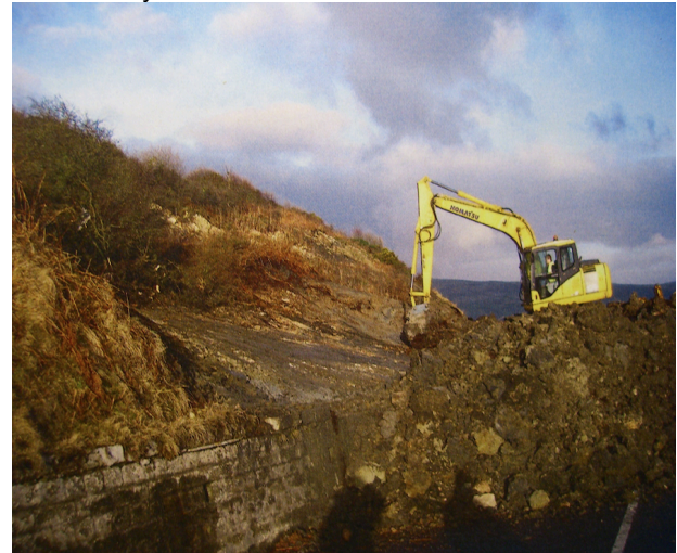
Figure 1 – Landslide debris on A2 Coast Road
