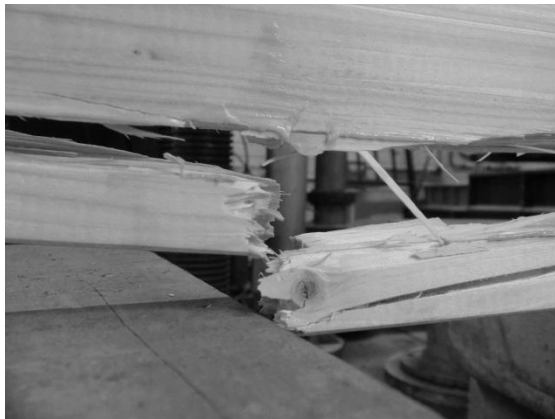
Fig. 14a Typical tensile failure of unreinforced glulam timber
