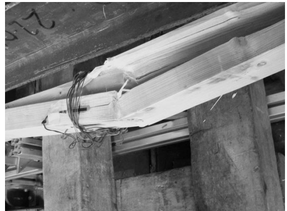
Fig. 14b Typical compressive/shear failure of post-tensioned glulam timber
