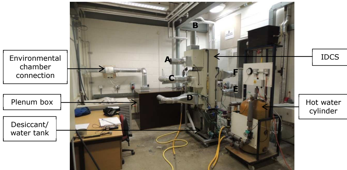
353 354 Figure 5 IDCS laboratory setup with labelled air flows 355
