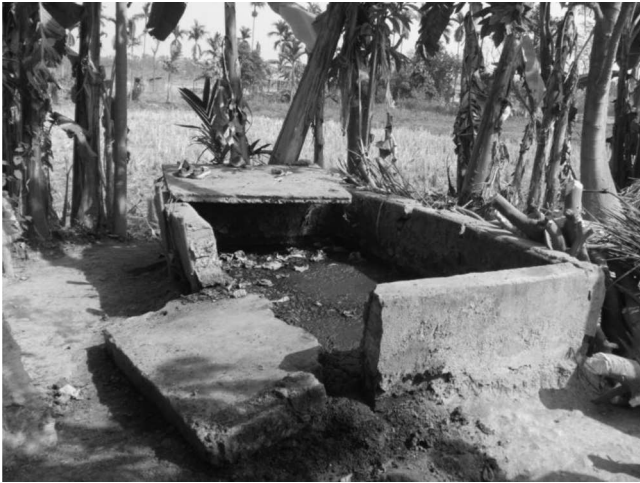
Fig. 2. Non-functional biogas unit at household number 12 (see Table 1) which has not been repaired for 6 months.
