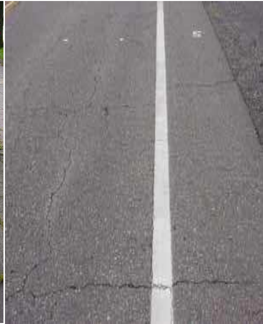
(b) Transverse Cracking
