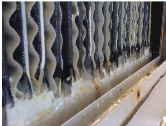
Figure 5-11 Dehumidifier HMX leakage in the IDCS
