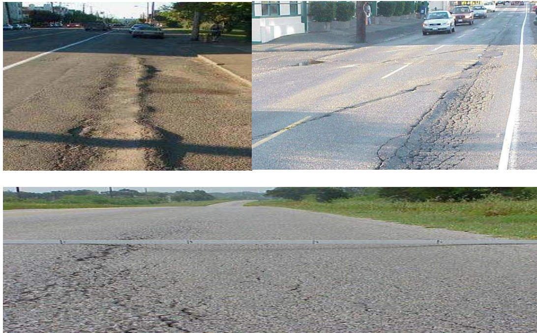
Figure 1.1 Permanent deformation in asphalt pavement (Science, 2014)
