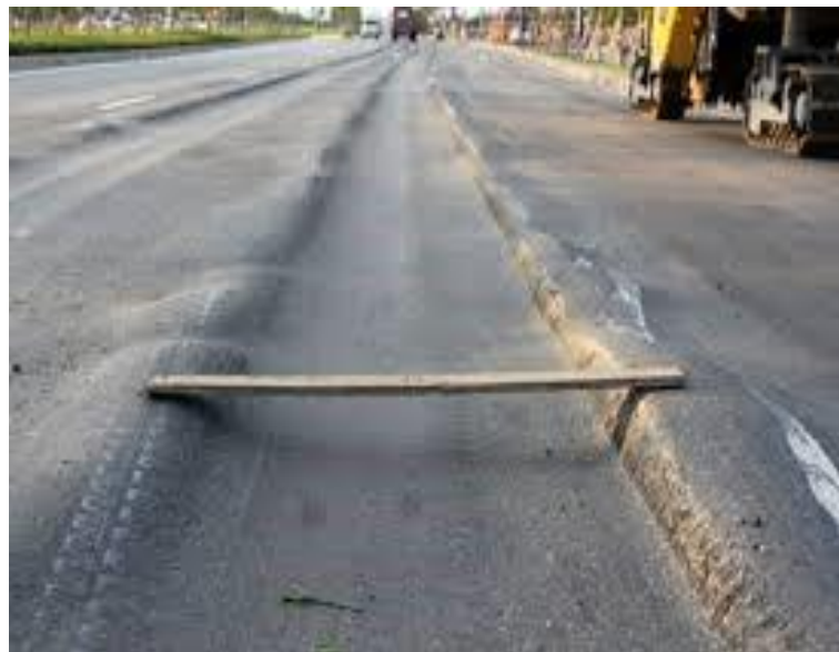
Figure 2.9: Rutting in practical engineering (Quang, 2014)
