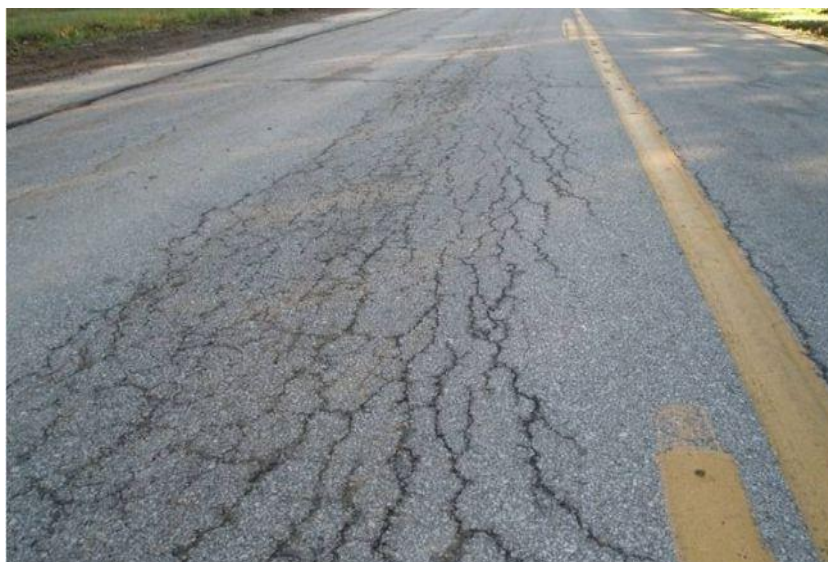
Figure 2.7: Fatigue cracking in practical engineering (Fatigue cracking, 2015)
