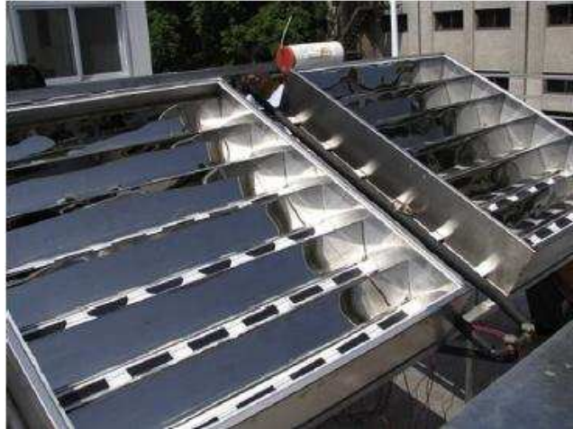
Figure 2.2.14 Illustration of CPVT mounted on the roof (Al-Alili et al., 2012)
