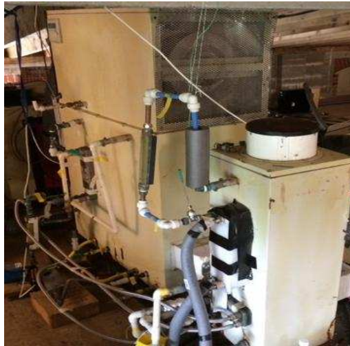
Figure 6.2.3 The dehumidifier and regeneration unit
