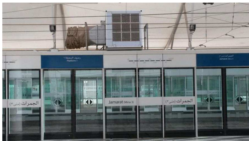
Figure 9.2 Evaporative cooler installed in Jamarat train station in Mina Valley
