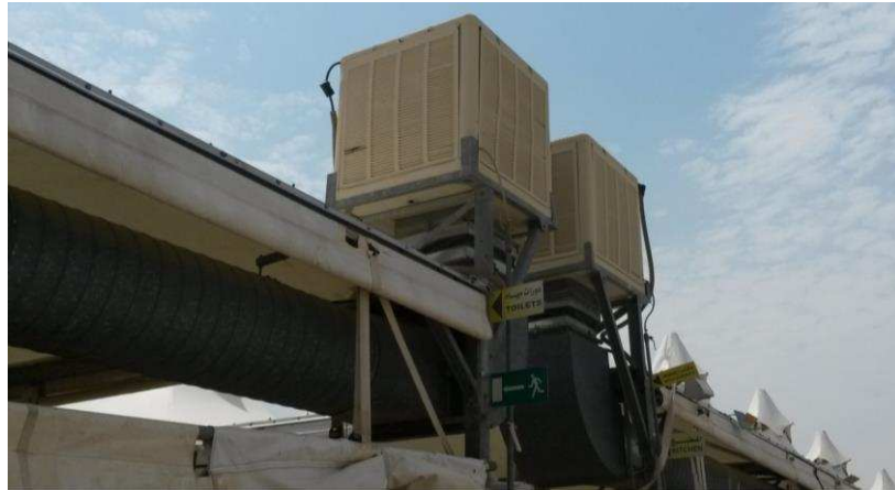
Figure 9.3 Evaporative cooler installed in Mina Valley
