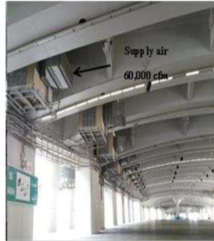
(b) Evaporative cooler unit
