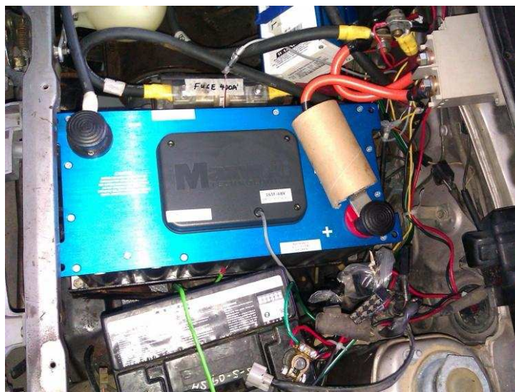
Fig 47: BMOD0165P048 installed just above the electric motor. Top right is the high current contactor which is activated by a 12V coil and a manual switch on the dashboard of the vehicle.
