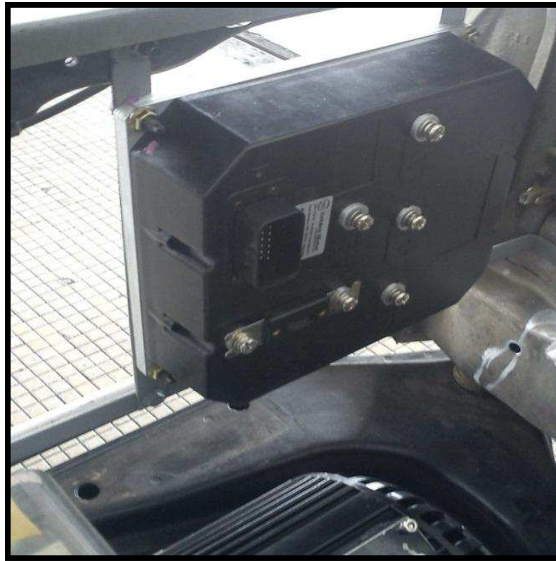
Fig 44: 500A Motor Controller successfully mounted in the same position as the radiator of a conventional vehicle
