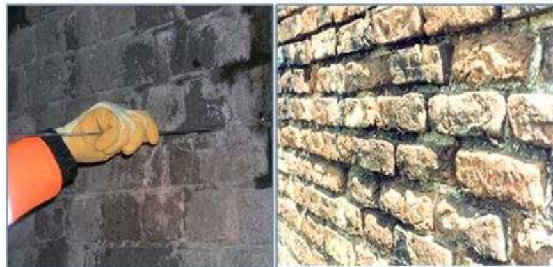
Figure 2.9 Open joints and weathered mortar (Courtesy of Network Rail Ltd.)
