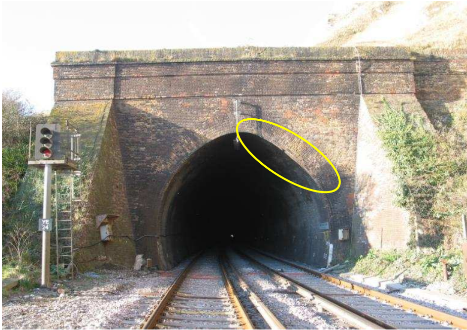
Figure 2.5 A typical tunnel deformation (Courtesy of Geodetic System Ltd.)
