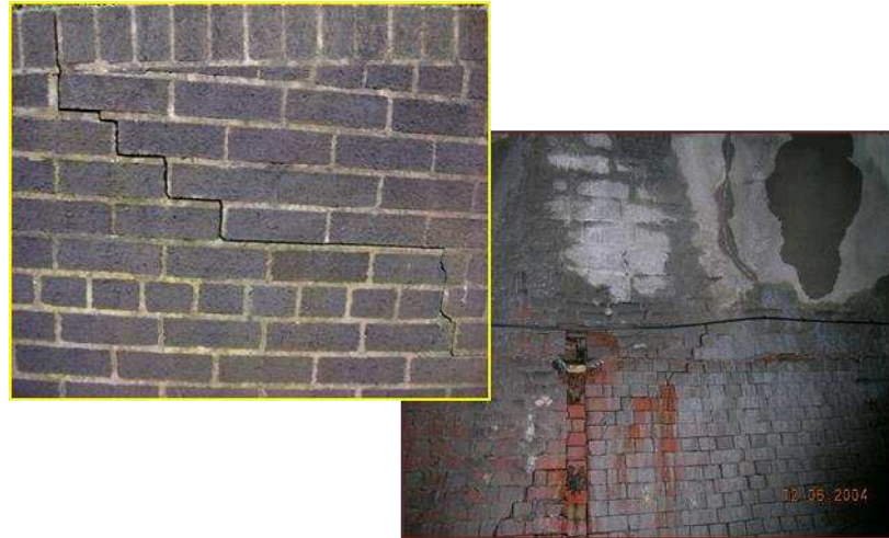
Figure 2.10 Cracks between bricks and mortars (Courtesy of Network Rail Ltd.)
