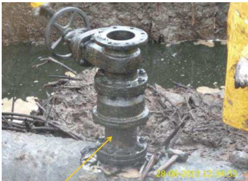
Plate 3-4: Arrow pointing at an illegal valve on a 28" pipe; picture taken on 28 th June 2013 (Shell Nigeria, 2013d).
