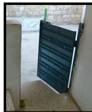
Figure 182: Metal door that is unsafe for children to use
