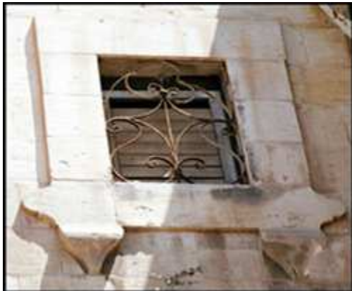
a) A square vent contains horizontal wooden blades, which have the ability to be opened and closed by changing the degree of the blades. It has an iron protection. Mengo's house, Nablus.
