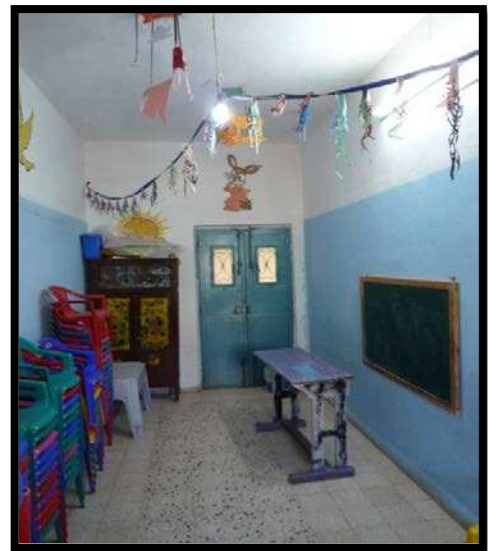
Figure 200: Photo shows the limited size of class No. 2, which has one window
