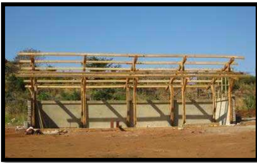
Figure 102: The toilet block consists of 4 separate sections: Adult toilets, girls and boys toilets and a store room with a sink (Holley, 2011).
