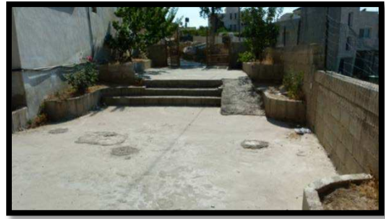
Figure 236: The opened out play area in two levels. This area has a ramp for moving goods to the facility
