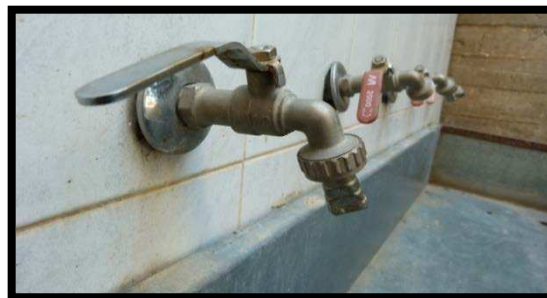
Figure 245: Destroyed water outlets for children's drinking
