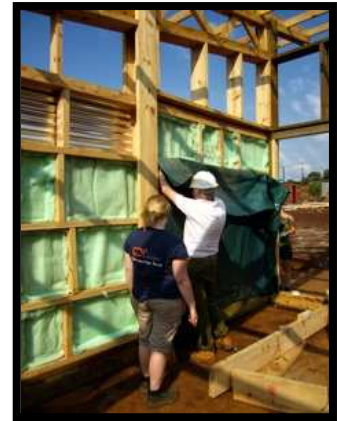
Figure 96: Fitting insulation and a deep proof membrane into the timber stud wall and an internal ply wood cladding (UoN, 2011).
