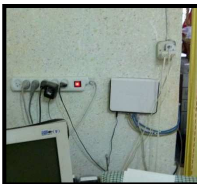
Figure 181: Overloaded plug sockets
