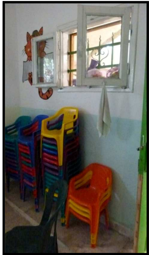
Figure 197: High windows that cannot enable children to view the outdoors
