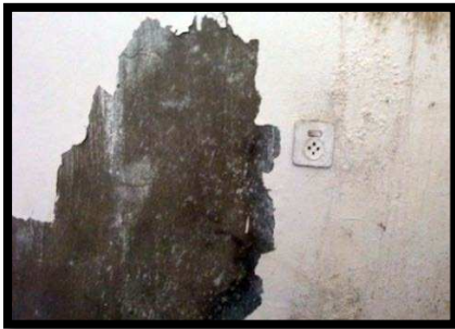
Figure 175: High humidity in the building
