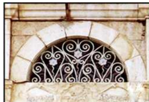
d) An arch vent, which is located above the main door, in Haddad's house has a floral metal decoration in the middle for protection, 1928.
