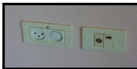
Figure 269: Some uncovered electric sockets in a low position
