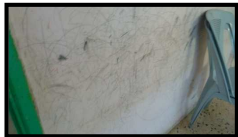
Figure 229: Dirty walls that need maintenance
