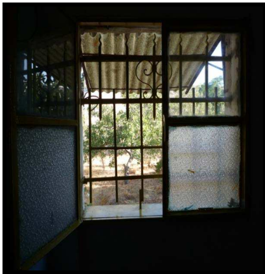
Figure 199: The only window that views the outdoor environment from inside the KG (Figure 80: C)
