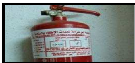
Figure 273: According to the label, this fire extinguisher should have been refilled in May 2008
