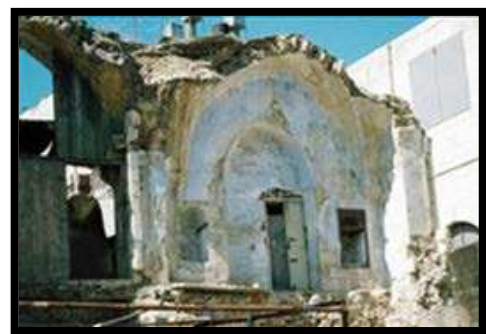
c) Section in a dome of a traditional house (type one), The old city, Nablus
