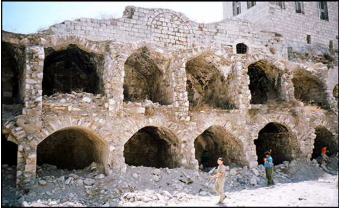
Figure 29: Section shows the building methods in a traditional building in PS. Nablus City.
