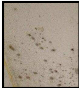
Figure 176: Mould on the KG lavatory ceiling
