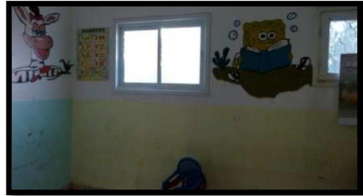
Figure 198: High windows that do not enable children to view and have contact with the outside environment
