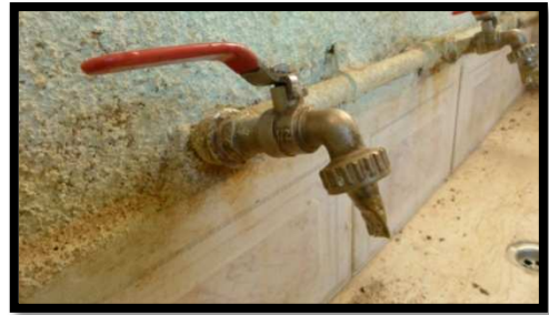
Figure 223: Unusable tap water for drinking
