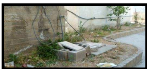
Figure 272: Pipes and dangerous materials
