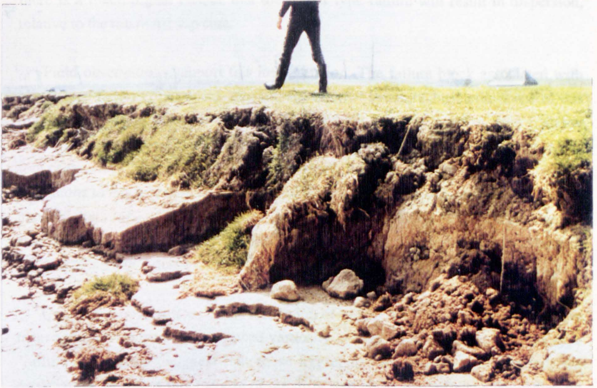
Plate 3.4 Disaggregated Blocks of Cohesive Bank Materials Following Mass Failure of IJssel River Banks, The Netherlands
