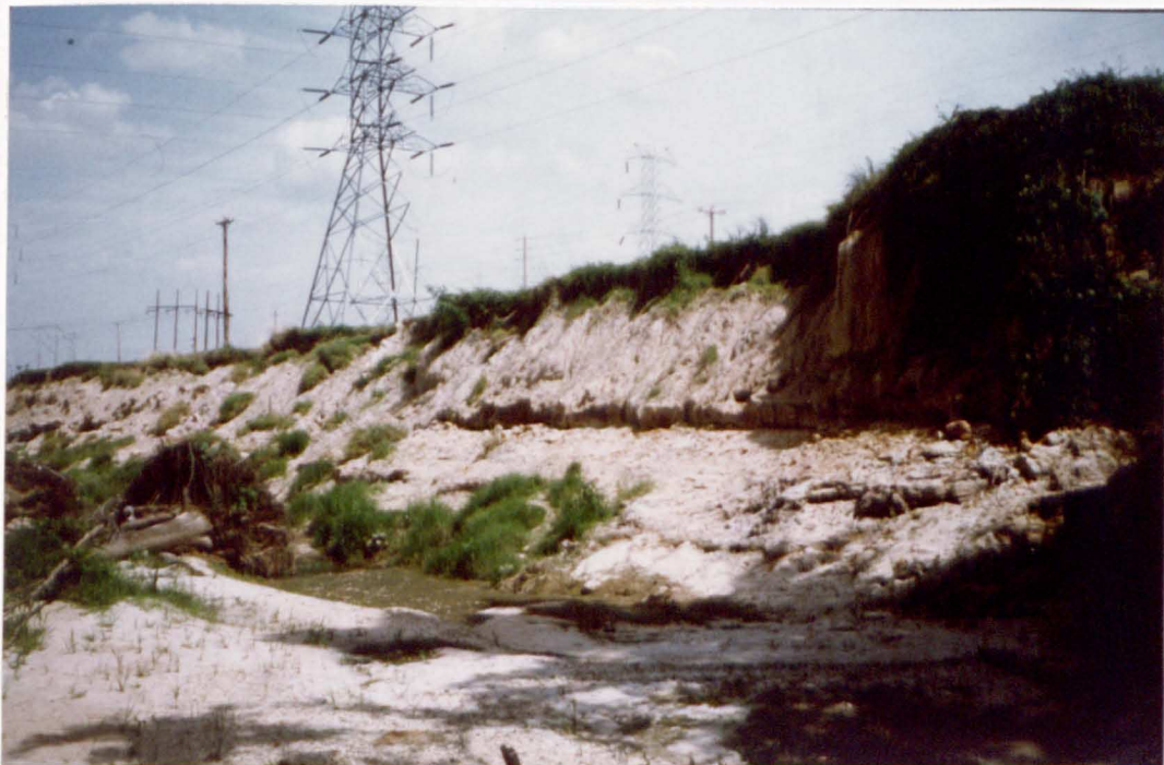
Plate 1.1 Power Pylon Under Threat From Bank Retreat, Nonconnah Creek, Memphis, Tennessee
