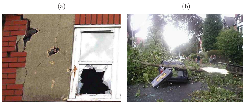
Figure 1.4: Damage to (a) building facades (Marshall and Robinson, 2006) and (b) cars due to windborne debris generated during the 2005 Birmingham Tornado (BBC, 2005).
