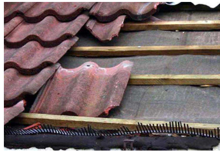
Figure 1.3: Photo from a damaged roof in Birmingham showing the typical UK roofing tile with nailing only at the top making bottom uplift easy (Marshall and Robinson, 2006).
