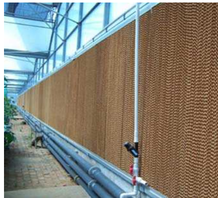
Fig. 2-11 Remote pad evaporative cooling system applied in greenhouse
