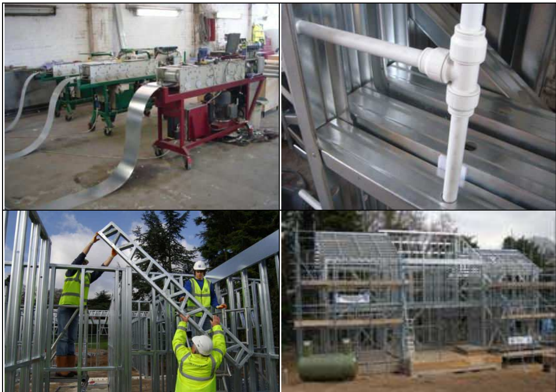
Figure 6-6: The Stoneguard House steel frame panels being prepared in the factory and installed on site with the help of undergraduate students of architecture (pictures by the author and by the photographer Robert Paulden)
