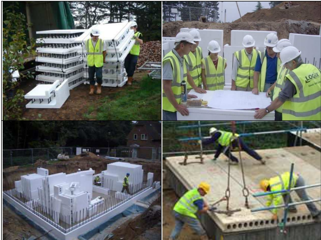
Figure 6-5: The construction of the Stoneguard house basement with help of undergraduate students of architecture (pictures by the author and by the photographer Robert Paulden)
