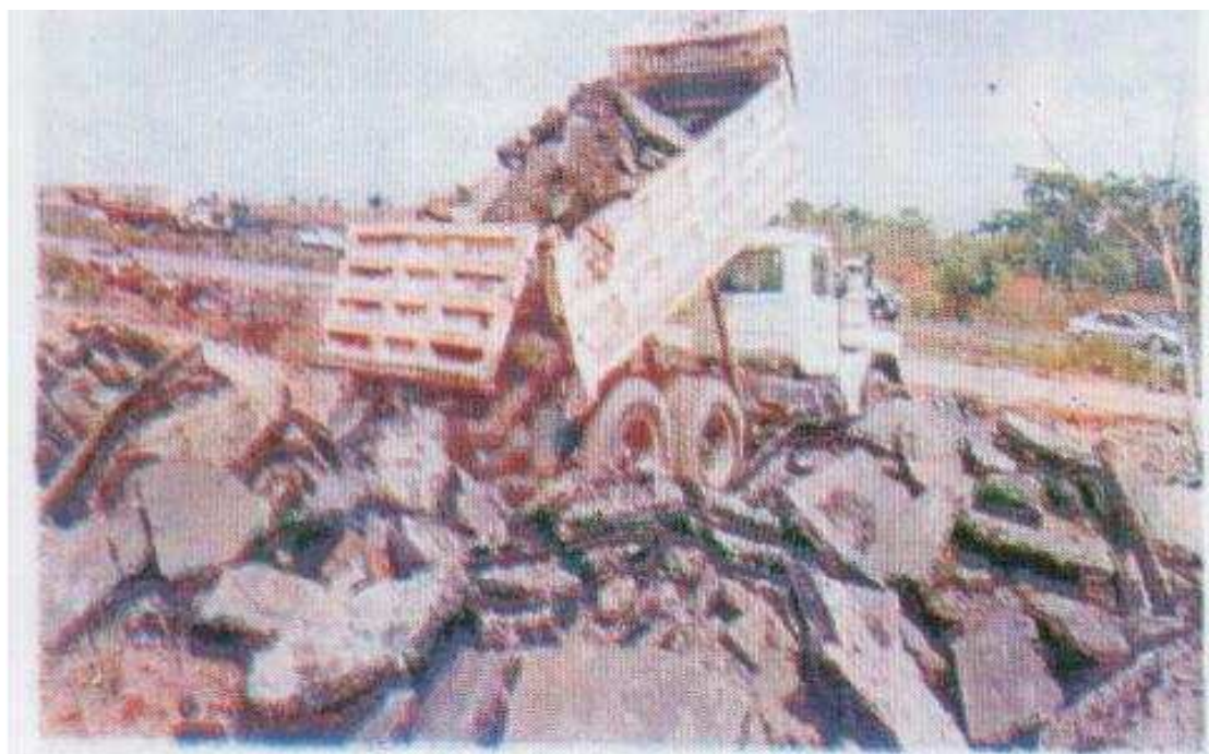
Figure 2.3b: Indiscriminate Dumping of Scarified Failed Pavement Materials in Nigeria (Eyo, 2005)
