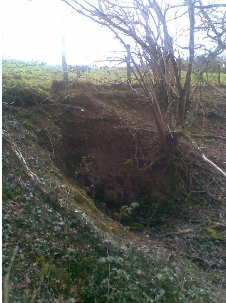
Figure 3.25 Local scour beneath a drain outflow on the lower Nant Melin-y-grûg.
