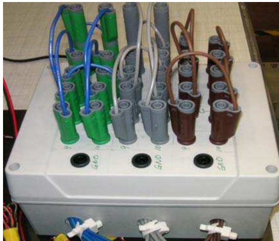
Fig. 5.17: Photograph of the switch box showing the interconnecting nodes and the bridge wires
