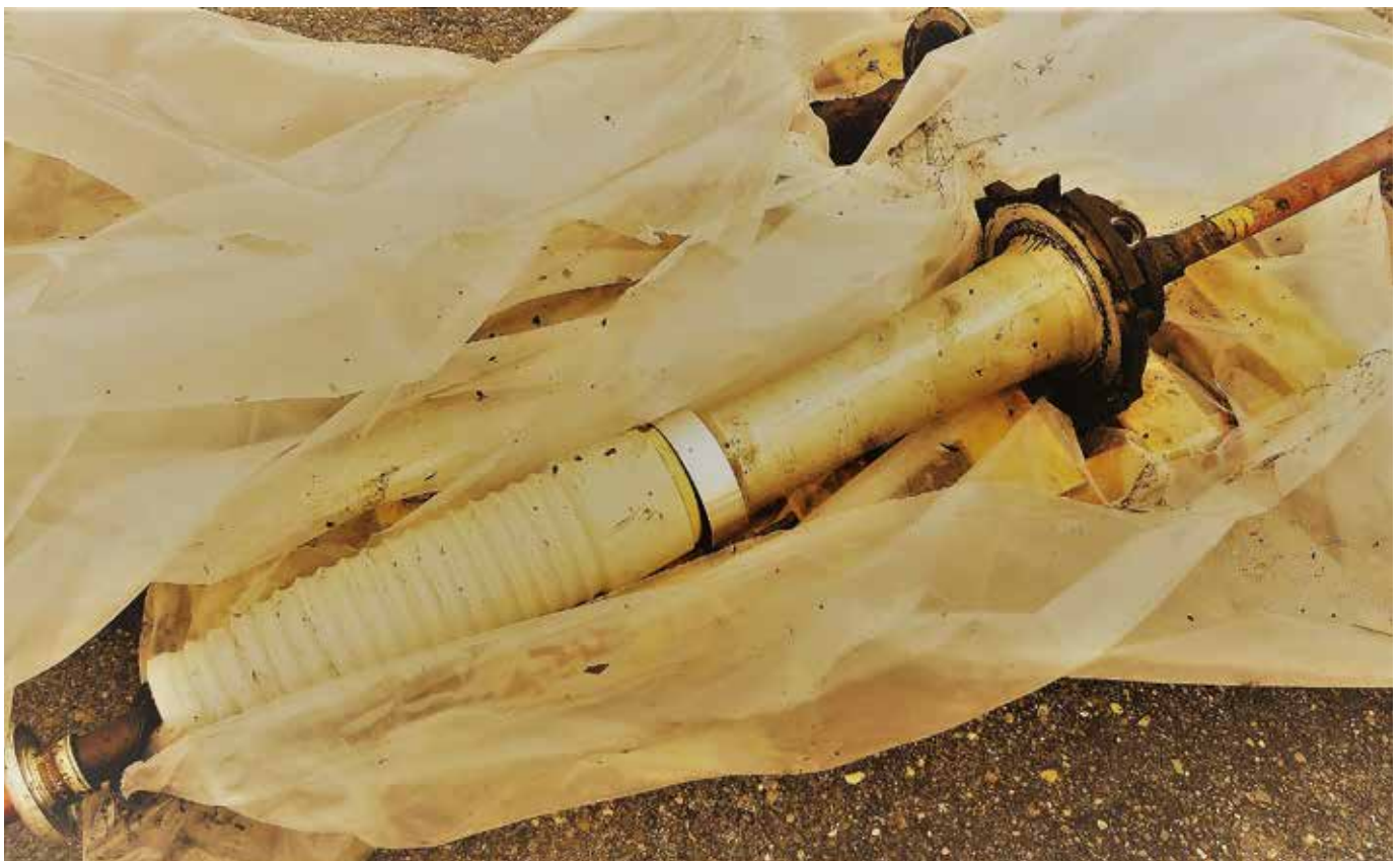
Figure 3. Investigated ABB, 69 kV, type O+C bushing failure for case study 2
