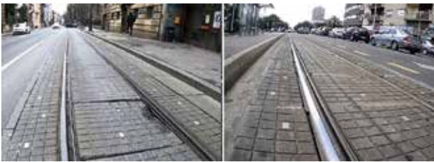
Figure 4. Reinforced concrete slab damage in track zone within a road system (left), deteriorated neoprene inserts next to rail web, absence of elastomeric sealing strip (right) [6]
