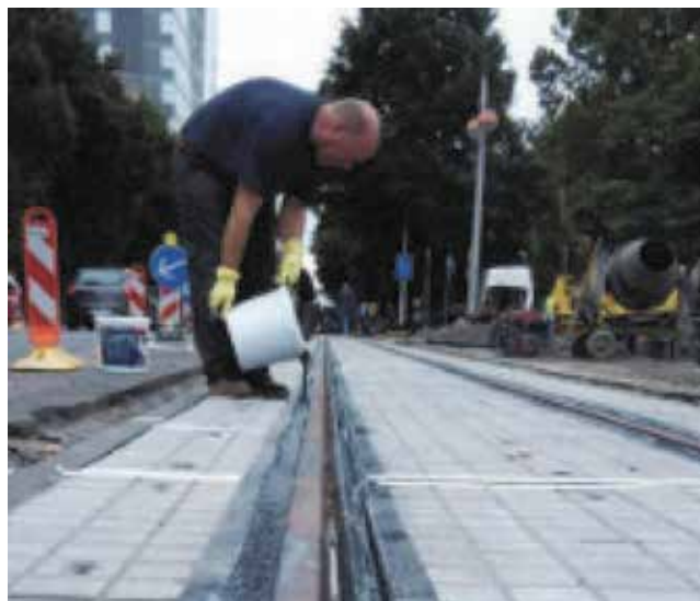
Figure 28. Placing fill material instead of sealing strips at Savska street tram section in Zagreb [9]
