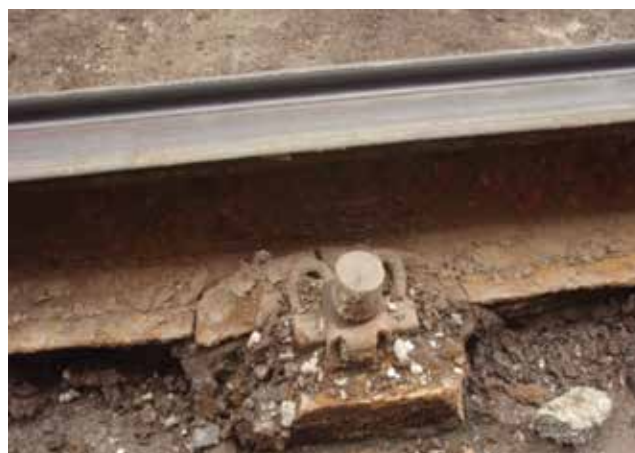
Figure 12. Rail foot rupture at fastening point on the street-running track
