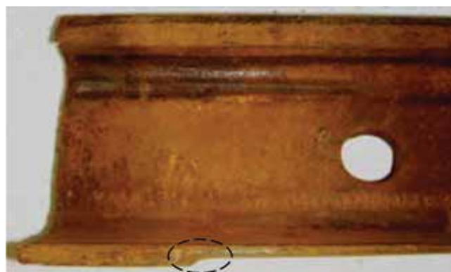
Figure 10. Tested sample of corroded rail, loss of material from the bottom side of the rail foot, circled points are the points of concentration of highest normal stresses [31]
