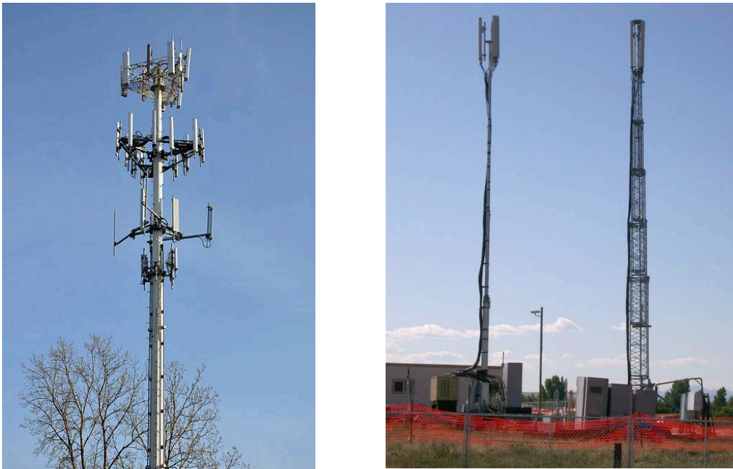
Figure 6: Cell tower / Cell on wheels
