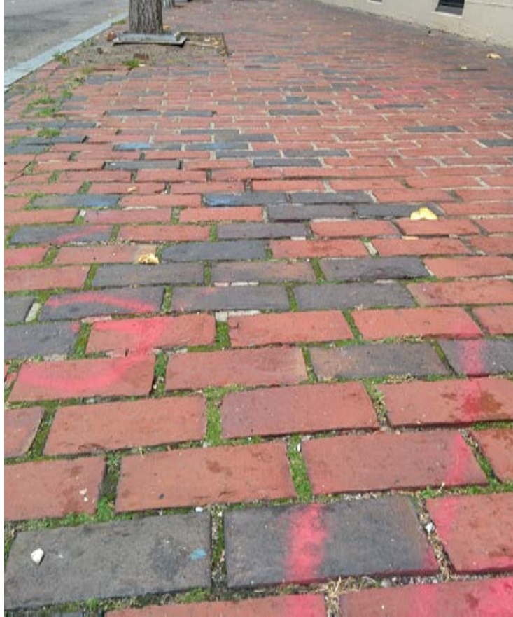
Figure 38: Close-up of community-based Surface 8
