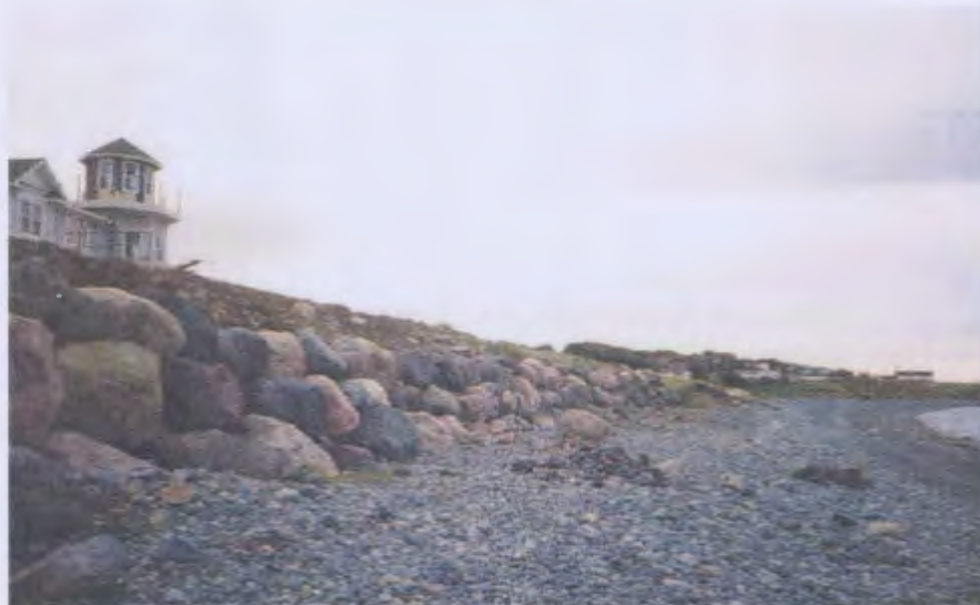
Plate 8.5: Boulder seawall constructed to halt erosion activity in segment 679 – 759 m. Note that the adjacent property is actively eroding and mitigation measures have not been put in place, potentially undermining the effectiveness of the seawall.
