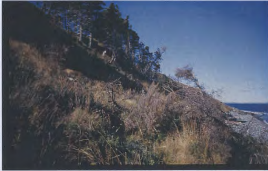
Plate 6.1: Photograph taken September 30, 2000 showing eroding slopes behind the Topsail United Church (segment 1702 – 1783 m). The Geological Survey of Canada established survey lines to monitor erosion rates at this location in July 1993.
