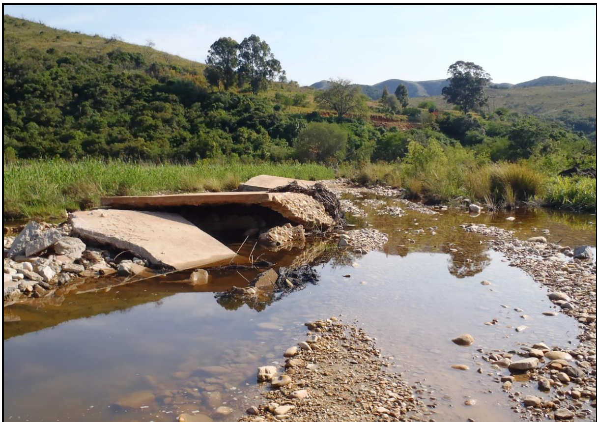
Figure 3.4 A low level bridge at the confluence of the Blindekloof stream and Kwa-Zunga River illustrating the extent of damage caused by the floodwaters during June 2011.
