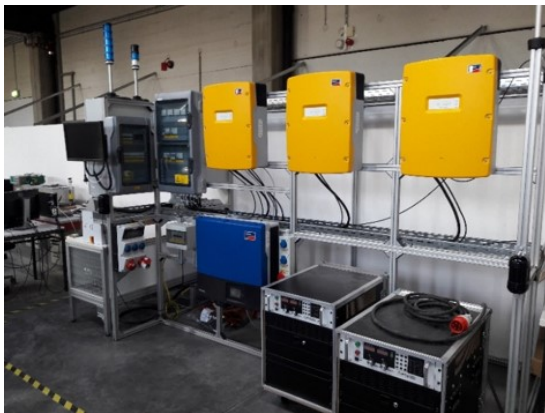
Figure 9.1: Electrical side of the BES.
