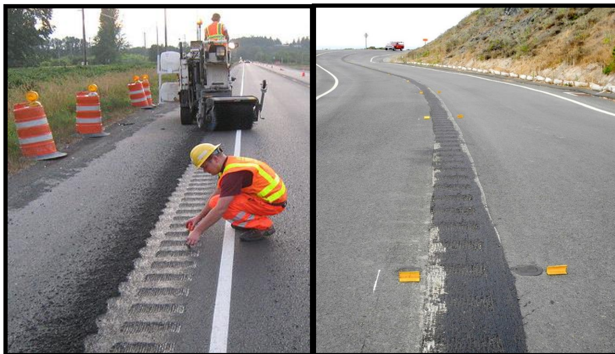
FIGURE 5. the installation of Shoulder Rumble Strip [left] and Centerline rumble strips [right]
