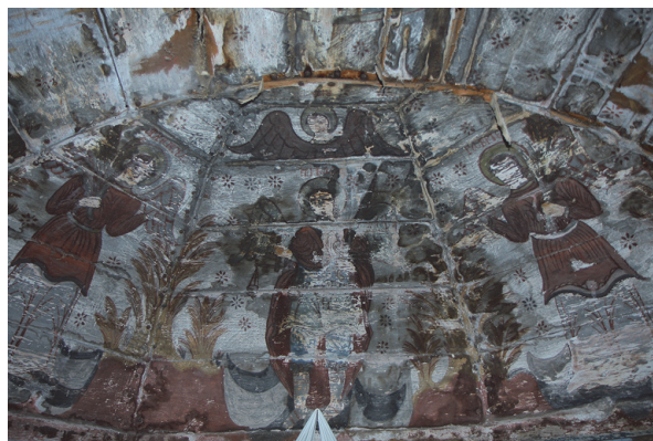
Figure 5. Semicap altar—degradation caused by humidity infiltration.
