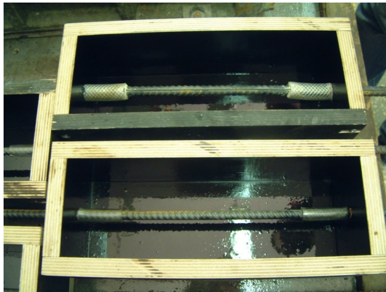
Figure 4.6: Reinforcing bars with sleeves at both ends, fitted into moulds prior to concrete casting
