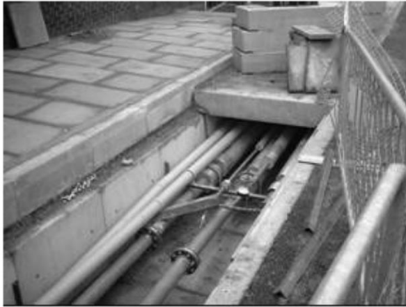
Figure 4-6: CHP pipes in a flush-fitting MUT at the University of Birmingham (Jefferson et al., 2006)
