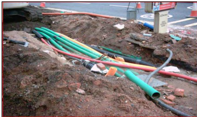
Figure 4-4: Utility placement within one of Eastside's 2m wide pedestrian walkways (Jefferson et al., 2006)
