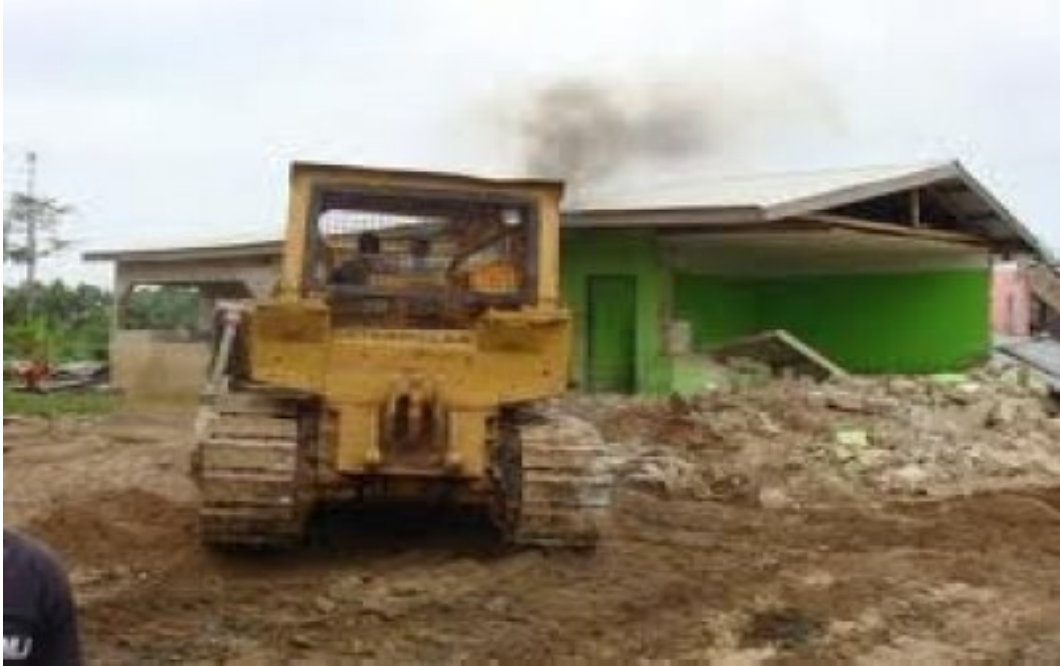
Figure 8.3: A brownfield site (Kumasi race course) being cleared to make way for redevelopment
