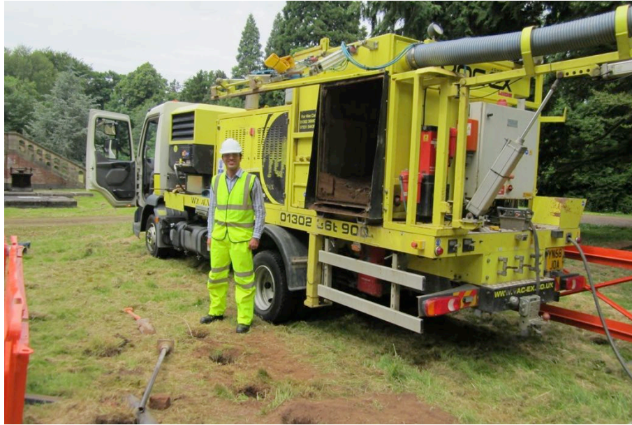
Figure 6.8 Vacuum excavator used for the trials at location "B" and the holes created for the RF tests.
