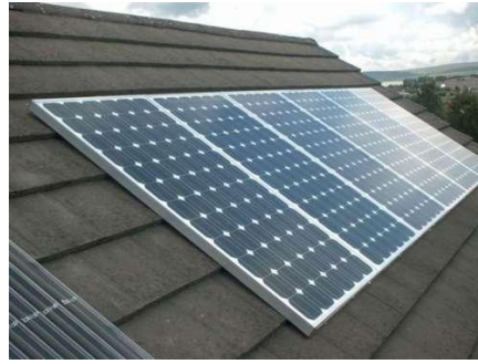
Figure 8.7: Photovoltaic Panels Reproduced from [210]
