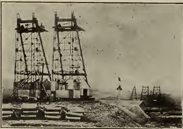
Fig. 1. Five Lidgerwood Cableways at Gatun Locks, Panama.
