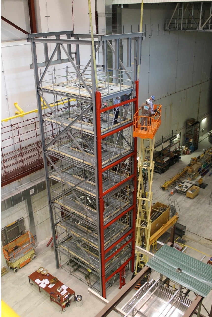
Figure 4.6: Phase 1 anode plane assembly (APA) installation frame (in red) being installed on the APA assembly tower at Ash River. In the foreground is the ProtoDUNE-SP trial assembly structure.
